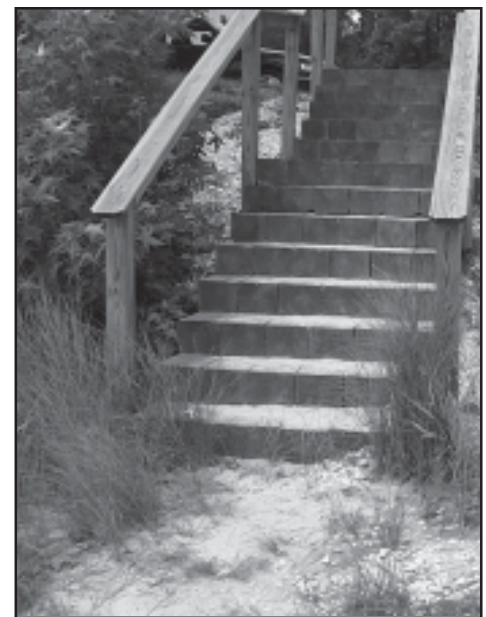
A wooden stairway may be the only feasible means of getting down a high bluff or steep slope.
